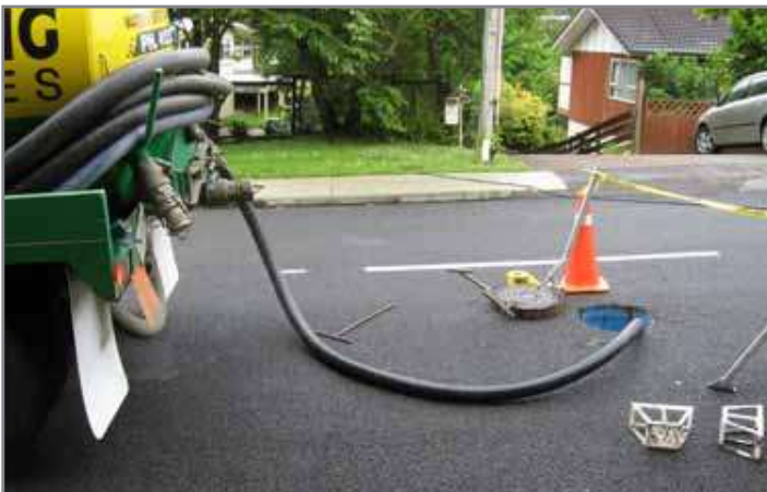
Fig.7 Sediment is removed from the sump with a vactor hose. Man entry is not required for this step.
