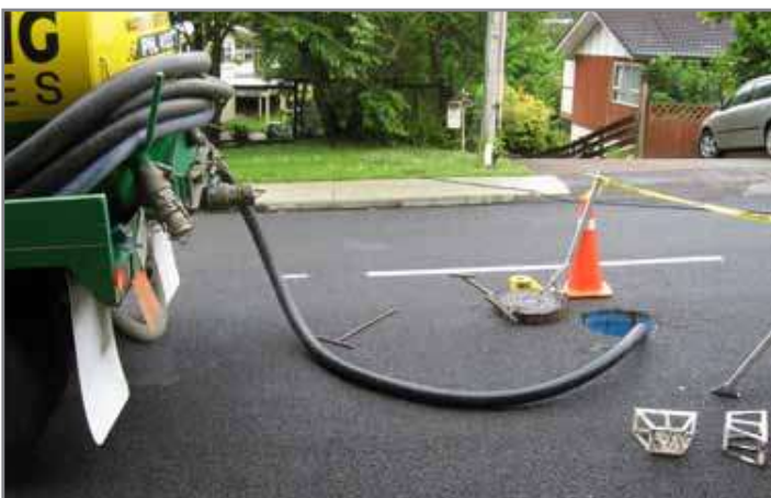
Fig.7 Sediment is removed from the sump with a vactor hose. Man entry is not required for this step.
