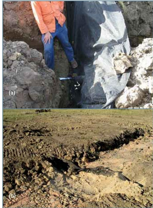
Figure 15. (a) Installation of sandblock perpendicular to a service trench. Note securing of geotextile to the optical fibre cable to prevent water flowing past the sand block. (b) Sandblock before final topsoiling.
